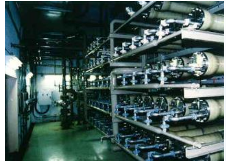
Sea water desalination plant (RO)
